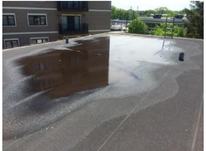
Standing water at roof edge. Recommend sweep roof, inspect seams and repair as necessary.
