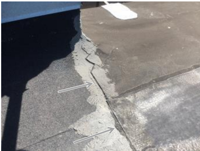
Seam failure at previous gutter edge repair at chimney area. This failure of adhesion appears to be due to lack of granular imbedding at the seam. Recommend repair seam, properly imbedding granulars in the process.
