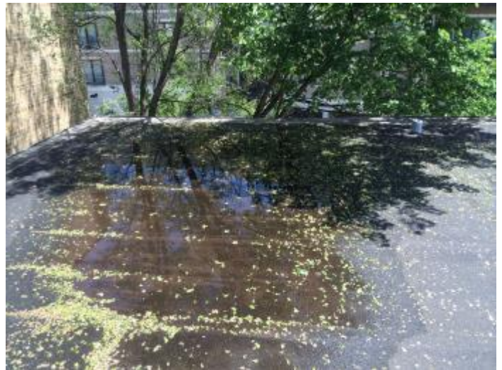
Standing water at roof edge. Recommend sweep roof, inspect seams and repair as necessary. In addition ensure tree is always pruned away from building to prevent damage to roof.
