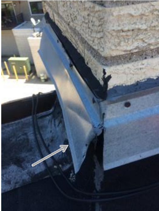
Metal chimney flashing damaged, and sealant cracked. Recommend replace loose flashing and apply new sealant.
