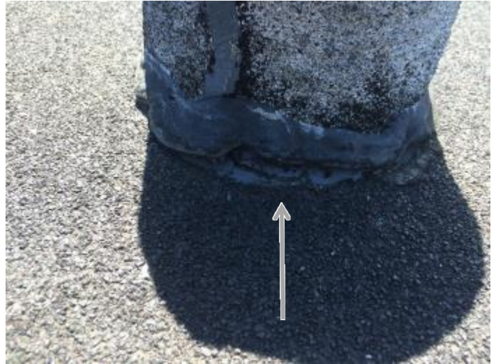
Shrinking or improperly applied sealant at base of pipe flashing. Recommend properly apply new sealant.
