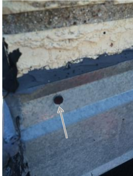
Exposed nails at metal chimney flashing. Nails are not the proper fastener for this application. Recommend replace improperly installed chimney flashing and apply new sealant.
