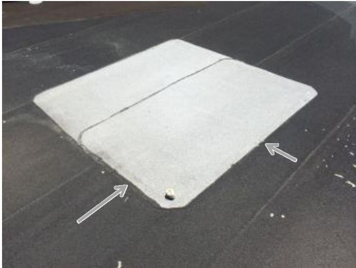
Previously installed roof patch. Recommend probe seams to ensure proper adhesion and repair as necessary.
