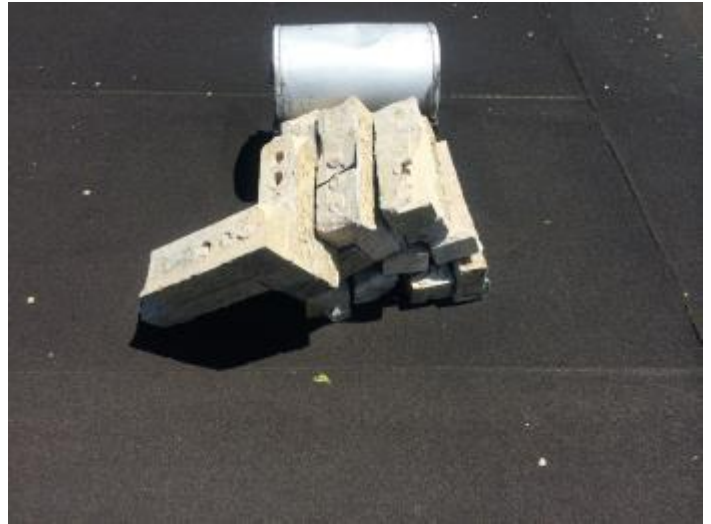
Debris left on roof. Recommend remove bricks and dispose.
