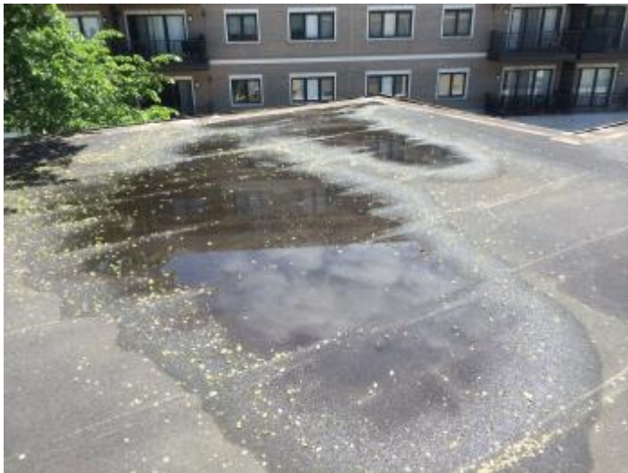
Standing water at roof edge. Recommend sweep roof, inspect seams and repair as necessary.
