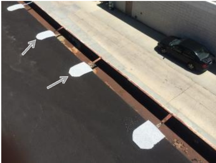
Previously installed repair at gutter edge.
