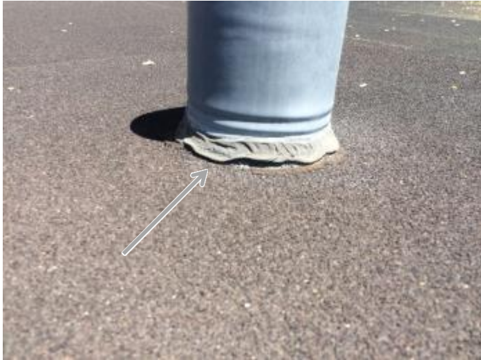
Shrinking or improperly applied sealant at base of pipe flashing. Recommend properly apply new sealant.
